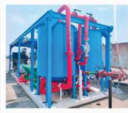
Sewage Treatment Unit
